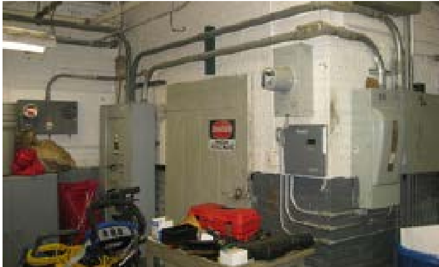
ONAWAY – SWITCH ROOM
