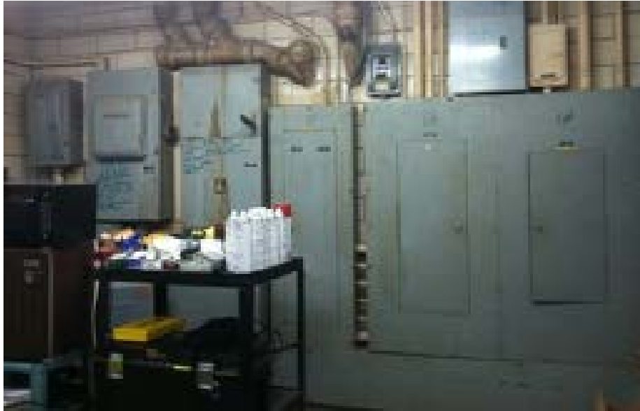
MERCER – PANEL BOARD
