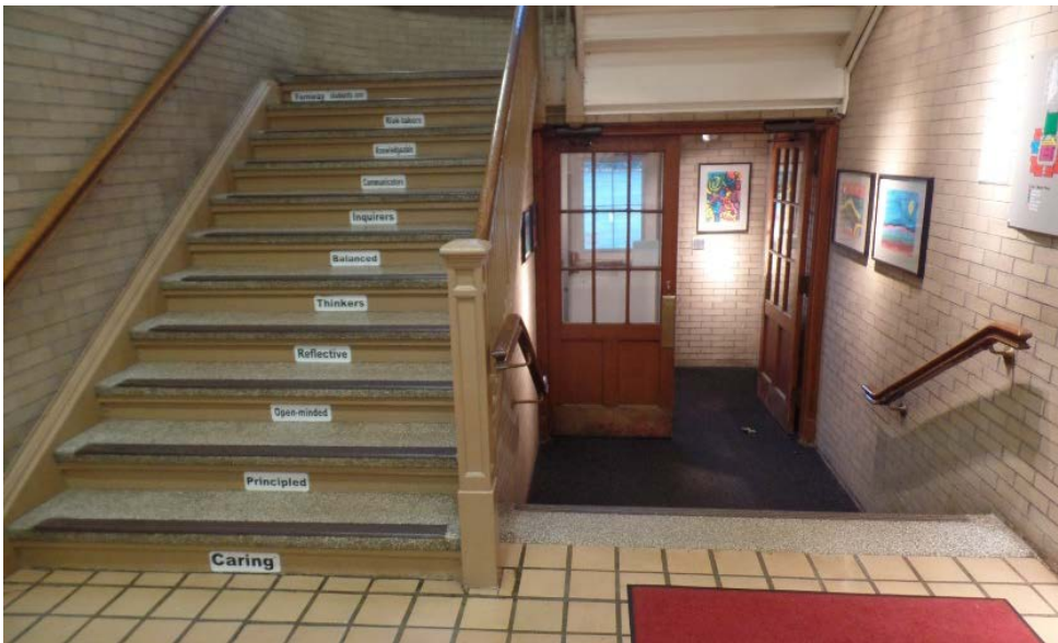
FERNWAY – INACCESSIBLE ENTRY
