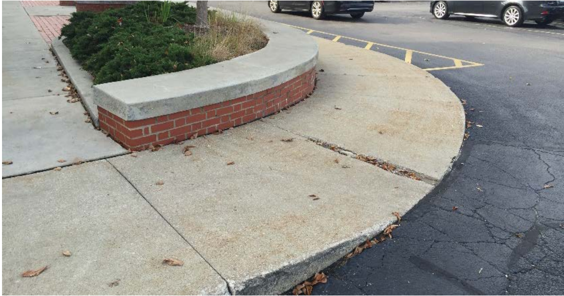
ONAWAY – NON-COMPLIANT CURB RAMP
