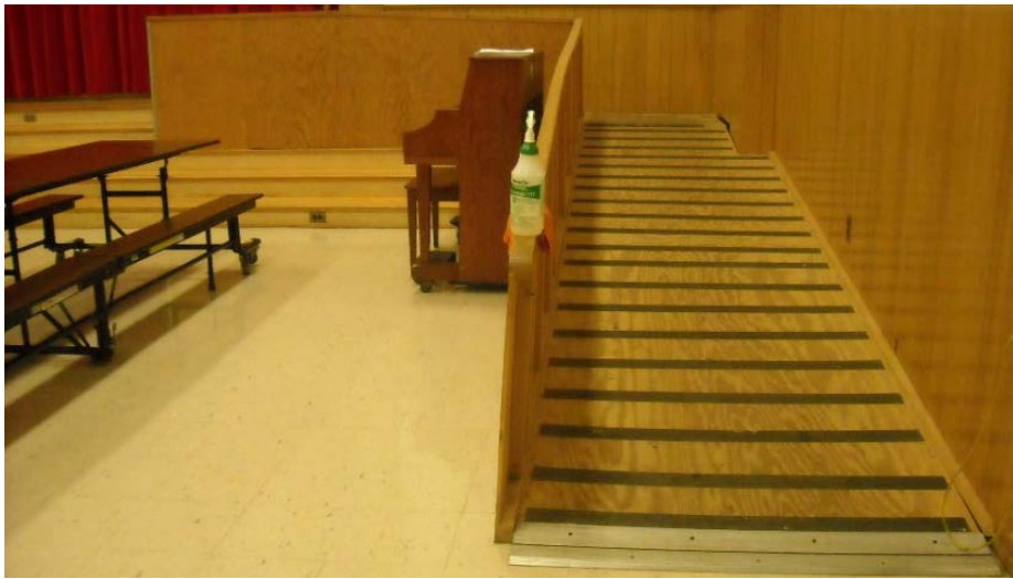
MERCER – NON-COMPLIANT STAGE RAMP
