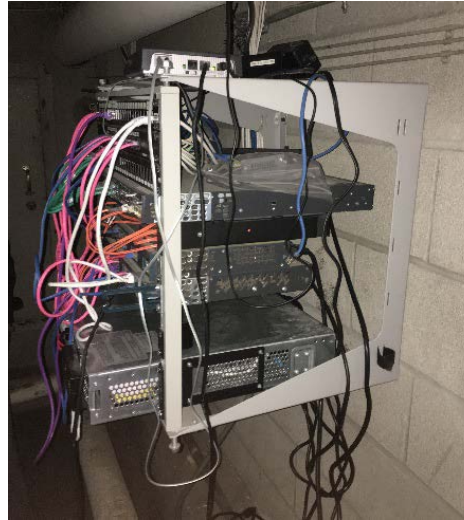
WOODBURY – RACK STORAGE
